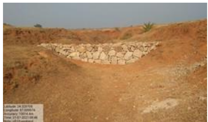
Loose Boulder Structure
